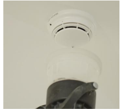
Figure 1: R.I Smoke alarm testing, fire alarm film
