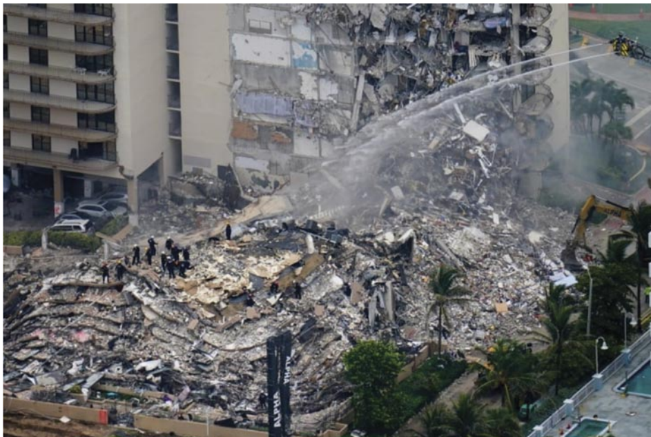
Champlain Towers Debris, CBC News, June 26, 2021 4 Canadians unaccounted for in wake of deadly Florida condo tower collapse | CBC News
