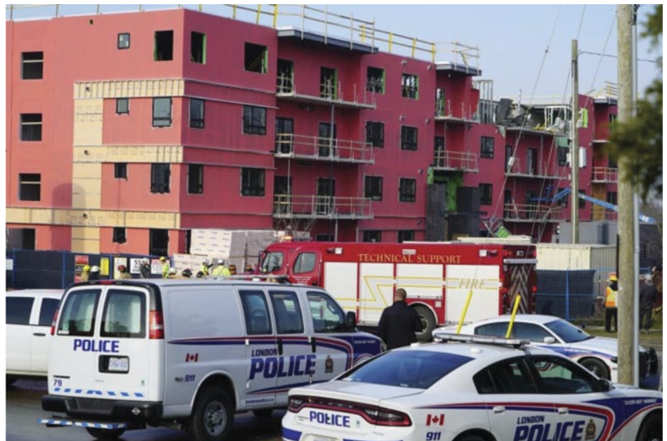
555 Teeple Terrace Partial Collapse, CBC News, Dec 11, 2020 2 dead, 4 in hospital after partial building collapse at London, Ont., construction site | CBC News
