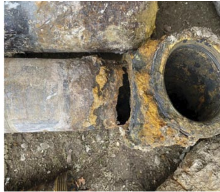
Corroding FDC pipe which was recently replaced.
