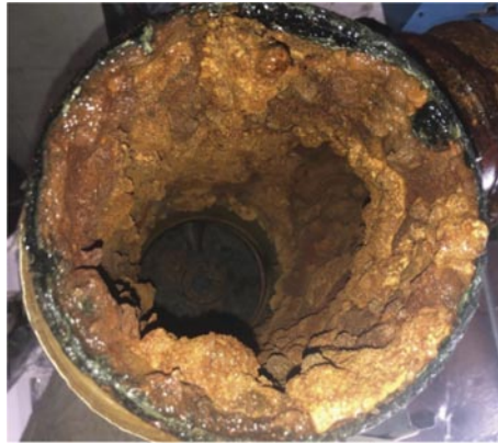
Internal piping on building side of the FDC check valve.
