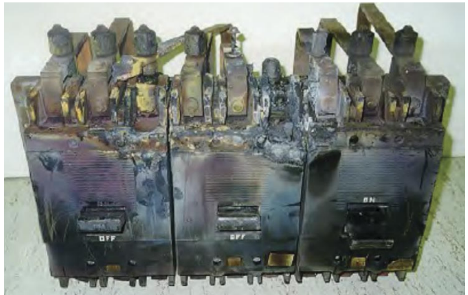
Figure 1 - Circuit Breaker Failure Caused by Surge Voltage 1
