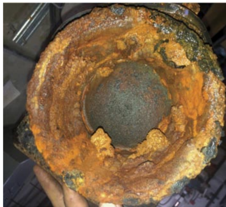
Internal condition of FDC check valve itself.
