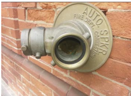
FDC hose connection point with its protective caps missing.
