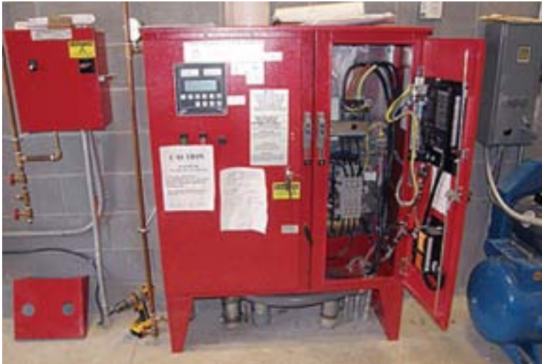
Electric fire pump controller with automatic transfer switch
