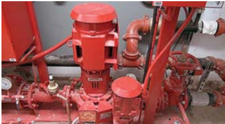
Electric vertical in-line fire pump
